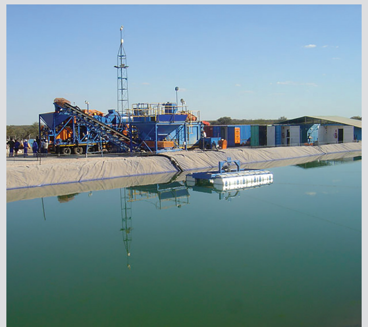
BK16 treatment plant
